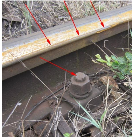
Fig. 3.2.2: First traces of derailment
