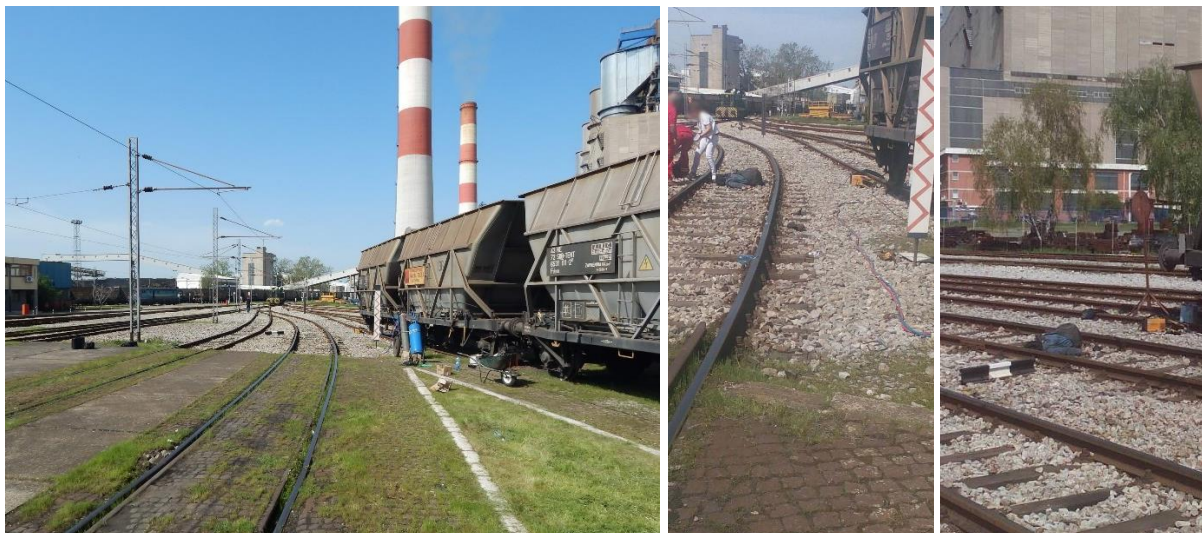
Figure 3.2.1: The appearance of the accident site where it came to overtaking of the loc. CEM-7 on the worker
