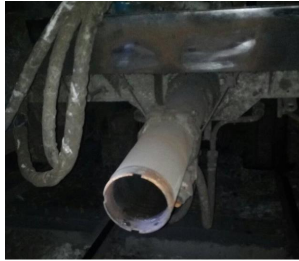
Figure 4.1.1.3: Appearance of a part of the decoupled coupling on the power car 412-061
